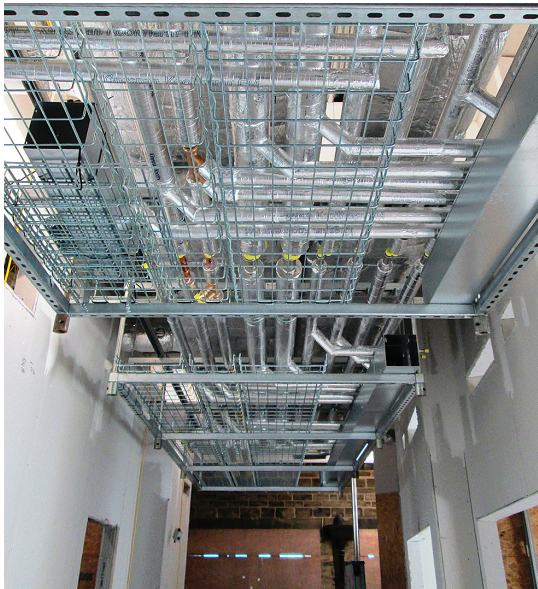
Figure 2 Ensure adequate provision is made to access above and around services to install penetration seals
