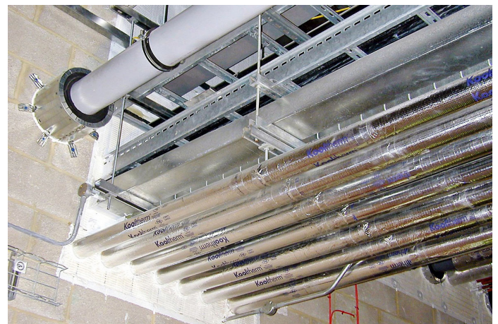
Figure 20 Multiple services within a single aperture. Lower services limit the access to the upper penetration seals
